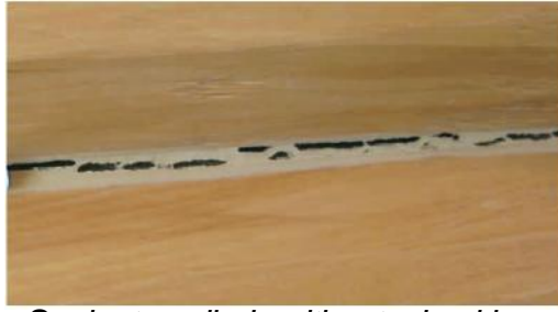
Sealant applied without a backing material to joint between unseasoned logs
