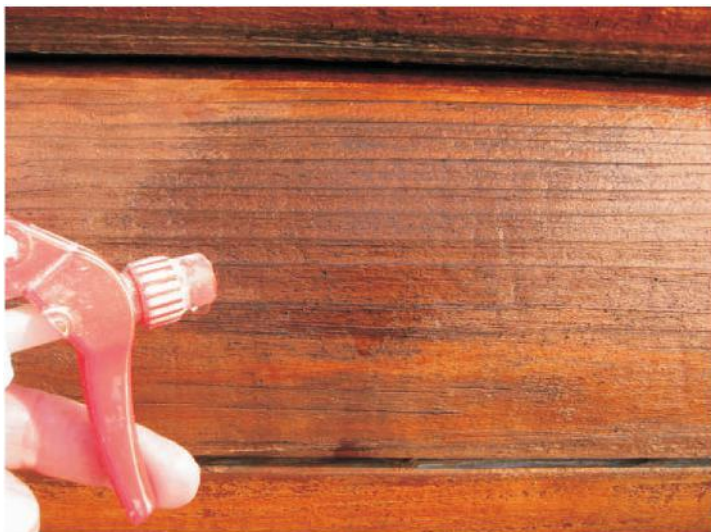
Water absorbing into wood through a finish that is no longer water repellent.
