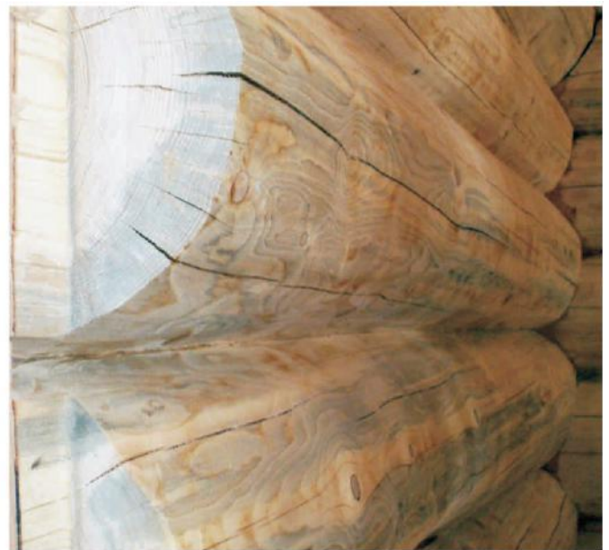
Blue stained logs in a wall
