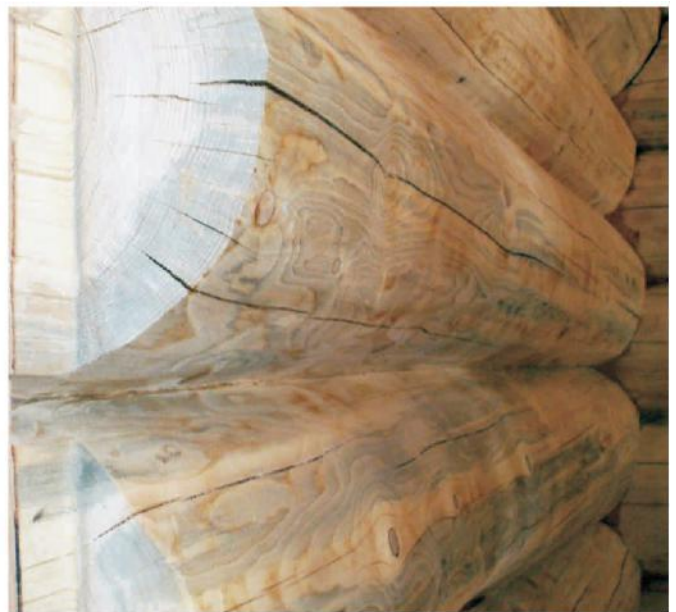
Blue stained logs in a wall
