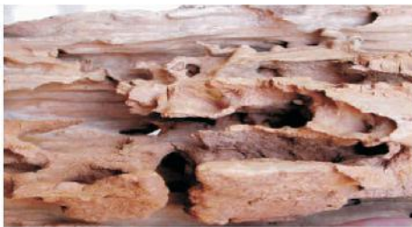
Carpenter Ant Damage
