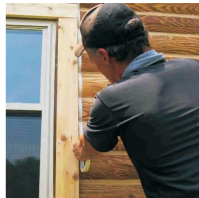
Apply masking tape to prevent sealant from smearing onto the adjacent logs.
