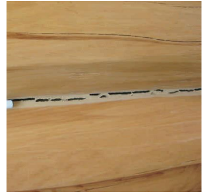
Sealant applied to a narrow seam without backing material.
