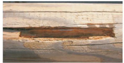
Cleaned out decayed pocket with some loose wood fibers.
