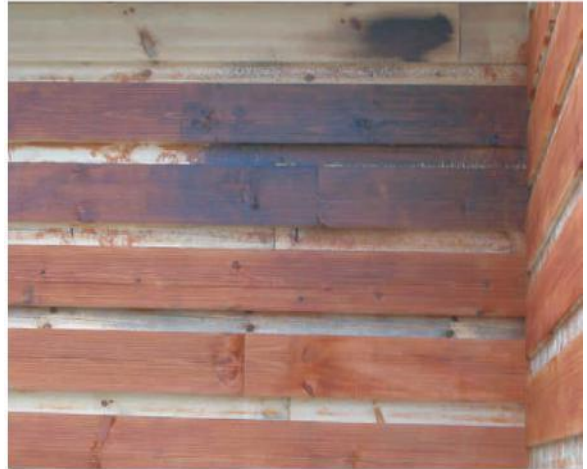
Inadequately mixed stain applied to wall.
