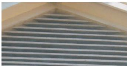
Hardware cloth over attic vent.
