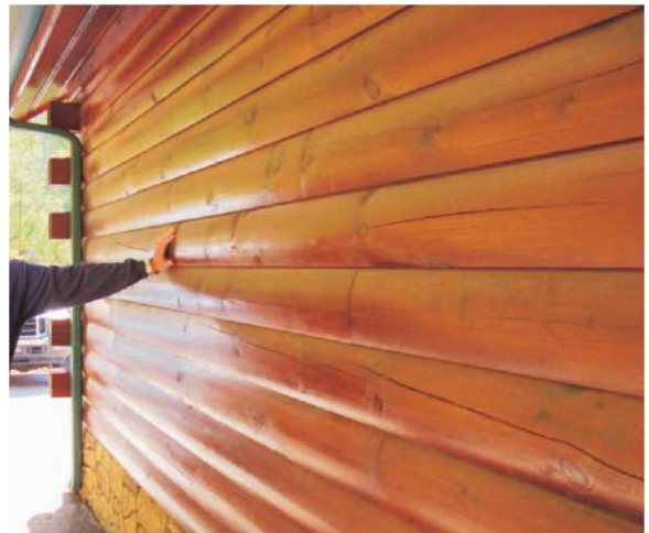
The same wall 6 years and 11 months later. No maintenance had been performed on the exterior finish during the intervening years.
