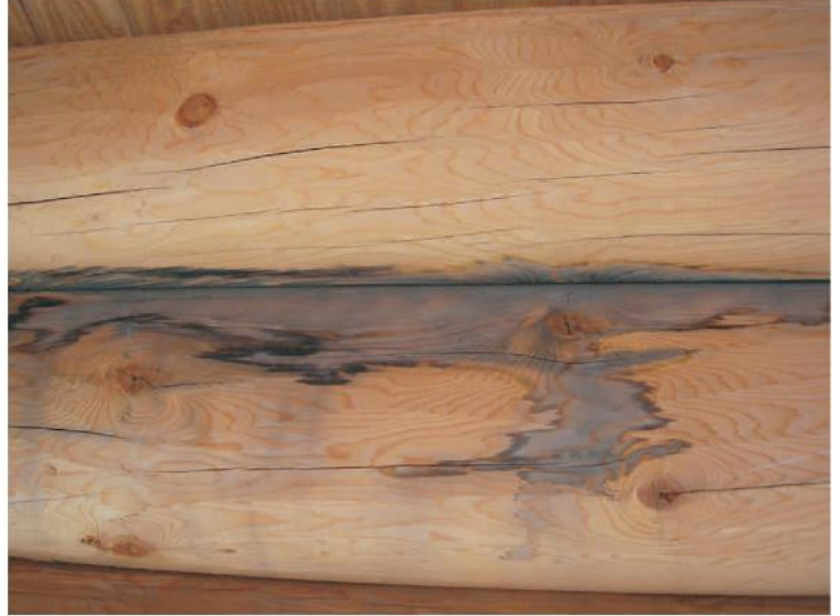
Interior Water Stains on Bare Wood
