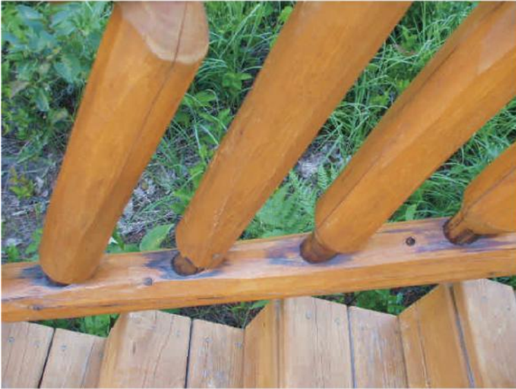
Exterior Water Stains Under the Finish
