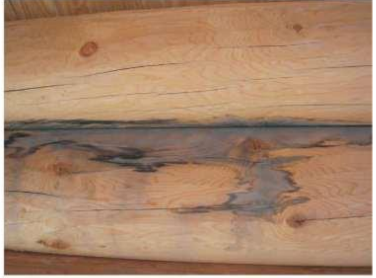
Interior Water Stains on Bare Wood
