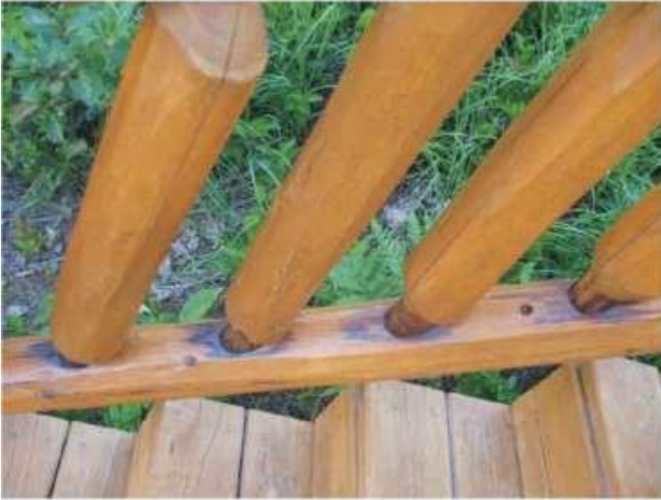
Exterior Water Stains Under the Finish
