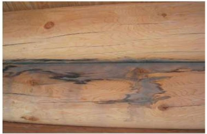
Interior water stains on bare wood.
