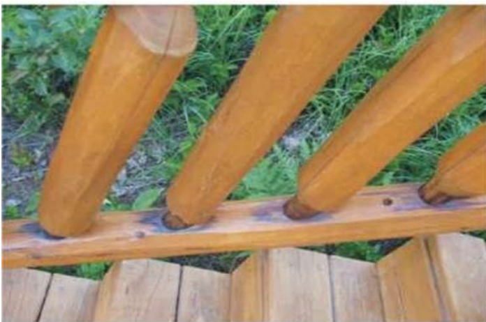
Exterior water stains under the finish.
